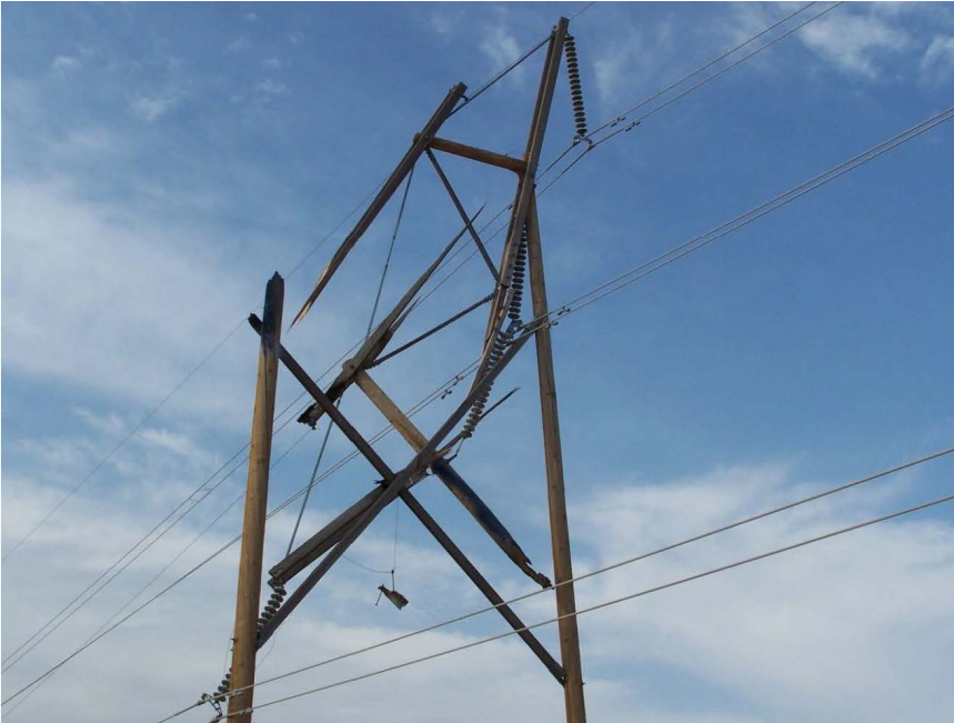
Fig 7 Structure Collapse Due to Fire Damage
