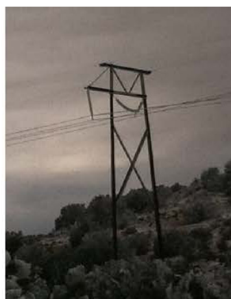
Figure 6 – Broken Structures due to Ice Storm
